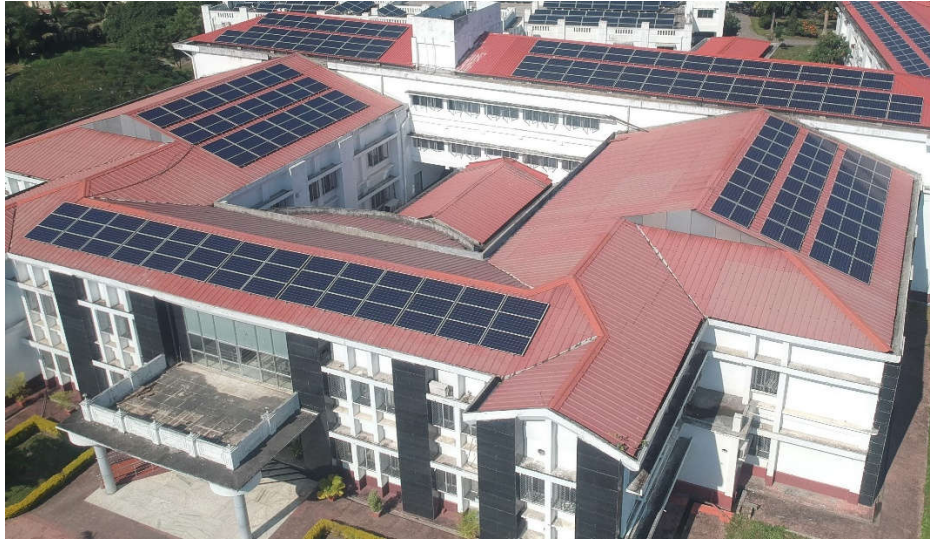
Fig 4 Solar power plant at University campus
